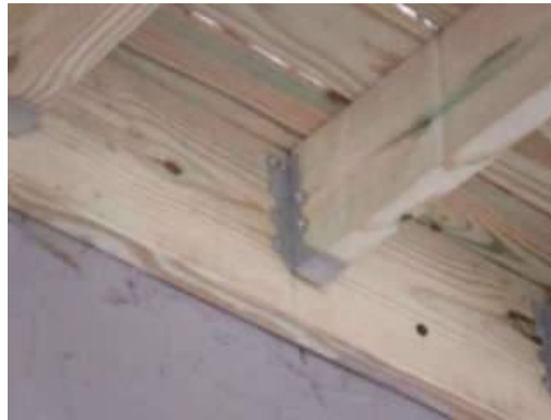
Photo 4-2 Deck bolt wrong size
