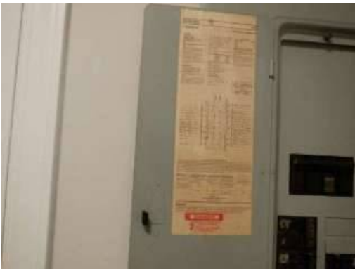
Photo 31-3 Main service panel Label Hard to read
