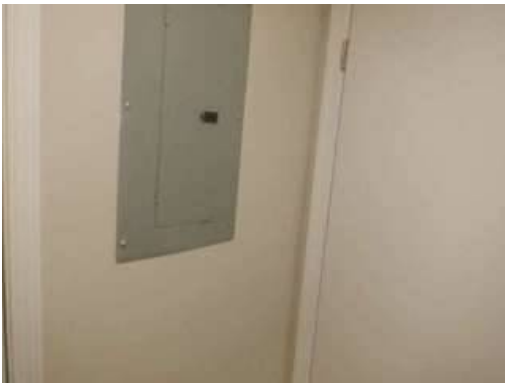
Photo 31-1 Main service panel
