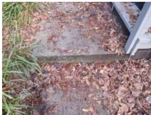
Photo 7-4 Possible Trip hazard
