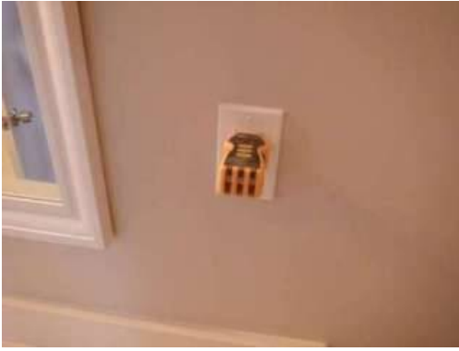
Photo 30-1 First-floor Bathroom GFCi Outlet not working
