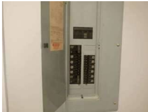
Photo 31-2 Main service panel
