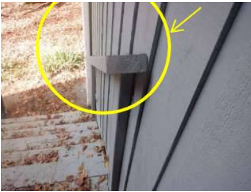
Photo 6-1 Handrail with no return
