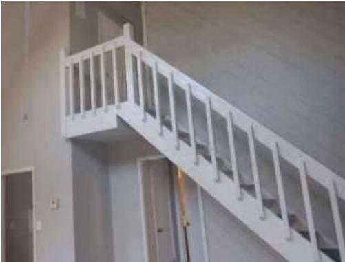
Photo 24-2 Guardrails should be 34"
