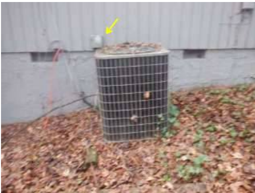
Photo 20-1 AC Conditioner blocking the fuse box
