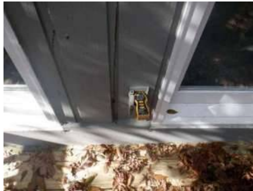
Photo 29-2 Deck GFCI outlet Not working
