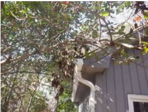
Photo 17-1 (R) side roof; tree limbs touching roof
